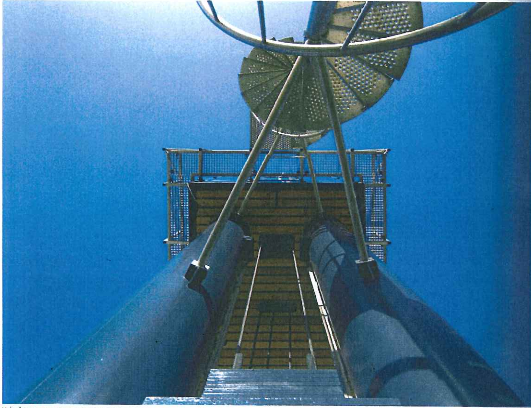
View from base towards engine room
